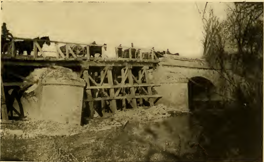
The bridge at Apremont, destroyed by the Germans and rebuilt by the American Engineers
